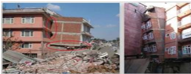
Fig1.1: 2015 Nepal Earthquake.Damages due to pounding effect
